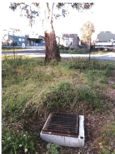
Existing stormwater pits and underground pipes running north-south to the east of the tree
